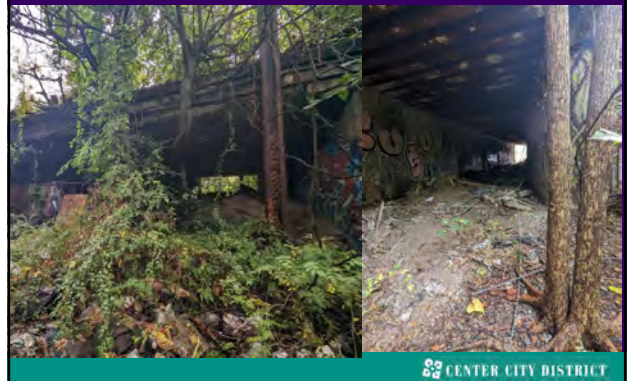
Scary sections under bridges
