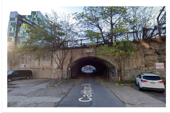
Figure 2 The Carlton Street bridge is 134' long with no functional lighting
