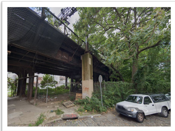
Figure 10 Netting along the viaduct prevents falling debris as the structure deteriorates
