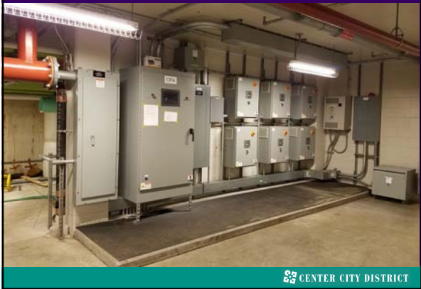
Maintenance of electrical systems supporting operations
