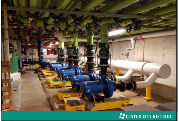
Plumbing systems for fountain & landscaping
